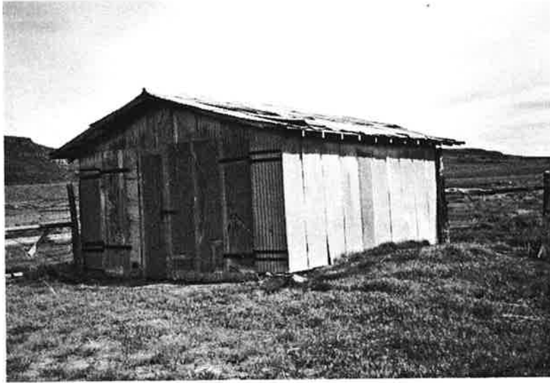
Garage, southeast view: ca. 1930; rectangular, one-story, stone foundation, wood frame, sheet metal siding. Low pitch gable roof covered with sheet metal. Door openings in north gable end, strap hinges. No windows. Good condition.
