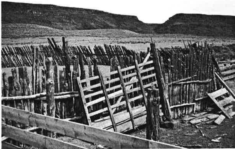
Corrals and Fences: Extensive system, variety of types and materials. Round corral constructed of vertical juniper posts set close together. Holding corrals, vertical juniper posts set several feet apart, with horizontal planks between. Rock wall (built ca. 1900), dry stacked rubble stone, several hundred yards long.
