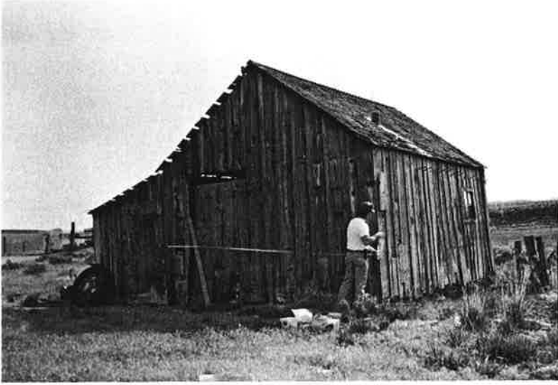
Blacksmith Shop, northwest view: ca. 1907; 20'x20'; rectangular, one-story, wood frame, vertical plank walls with exterior batts. Medium gable roof, wood shingle, lean-to on west elevation. Dry stone foundation. Small, 4-light window in east elevation. Two vertical plank doors offset center in south (gable end) elevation, Z-bracing, falling off hinges. Exterior siding warped and deteriorating. Roof materials missing. Fair condition.
