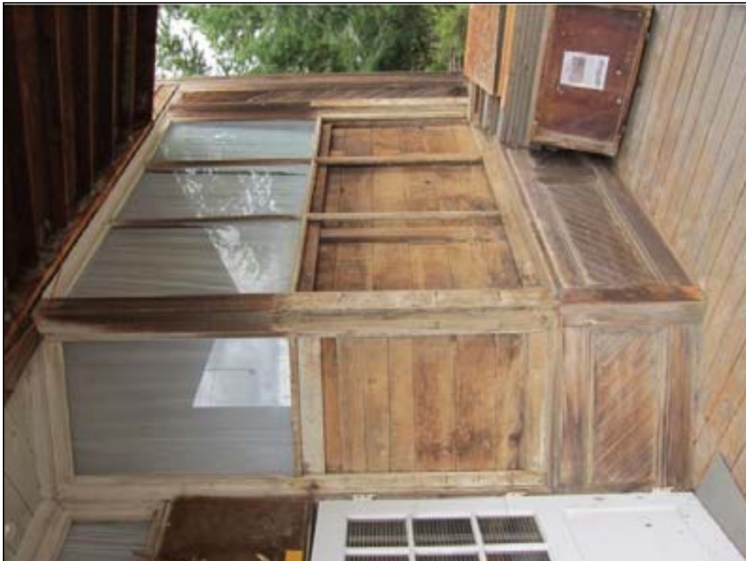
Photo 4 of 16: (OR_MorrowCounty_HardmanIOOLodge_0004) East façade looking north at a close up of the storefront windows and bulkhead.
